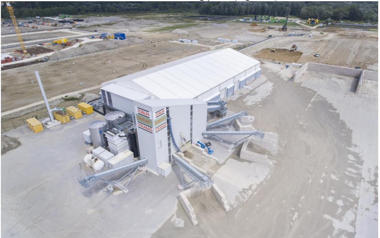
Figure 2: Areal view of the soil washing plant (front), sludge treatment facility (left hand side) and the reception hall (in the back). Copyright: ARGE AUDI IN-Campus GbR.
