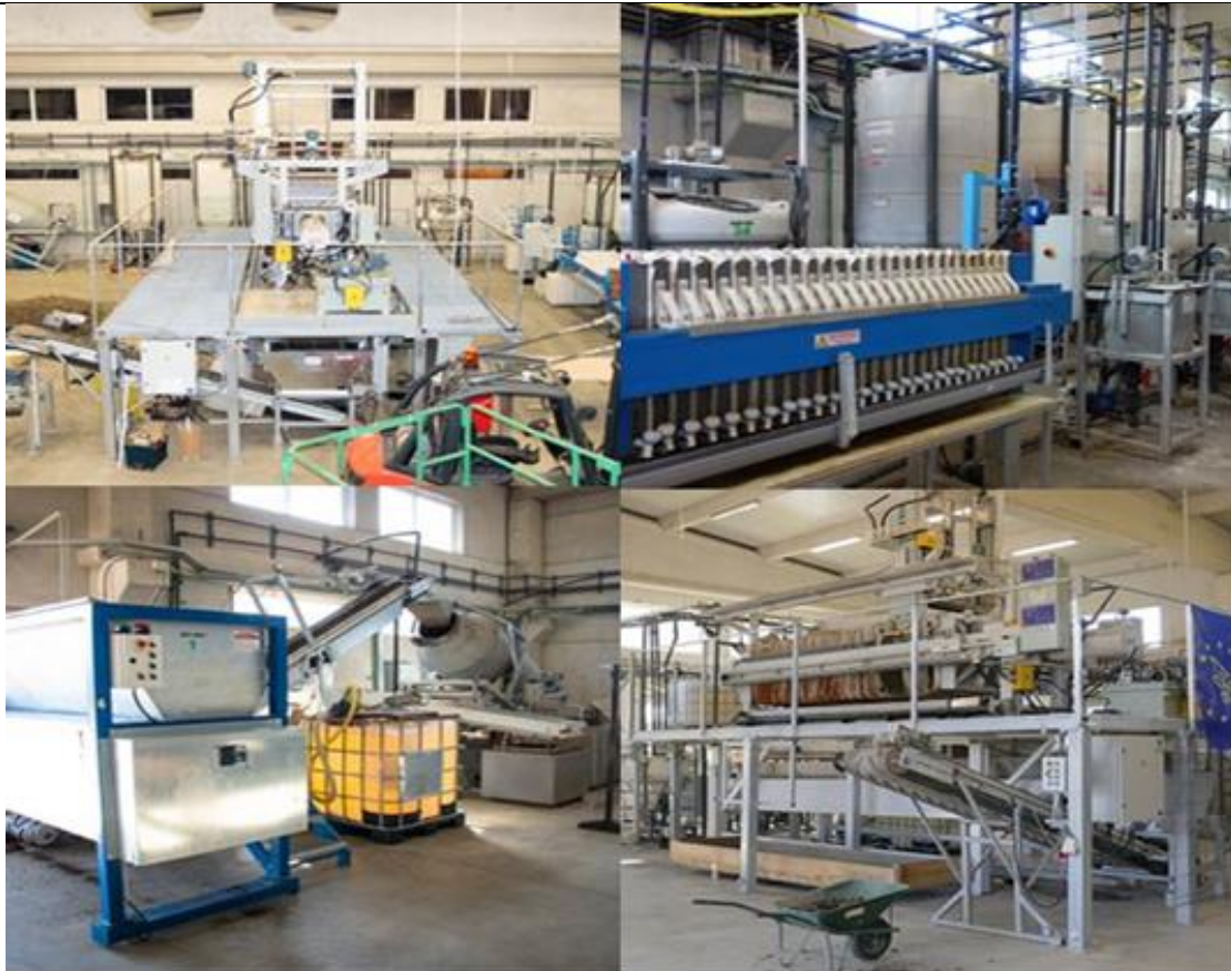
Figure 7: Stationary ReSoil® facility with capacity of 6 t/day constructed under LIFE+ programme .
