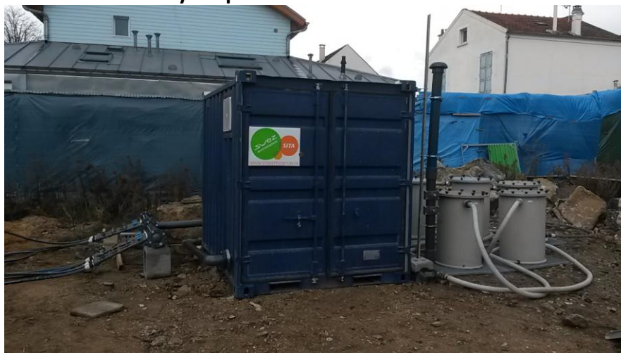
Photograph of SVE treatment facilities
