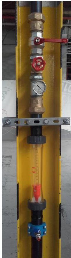
Examples of instruments along each extraction line
