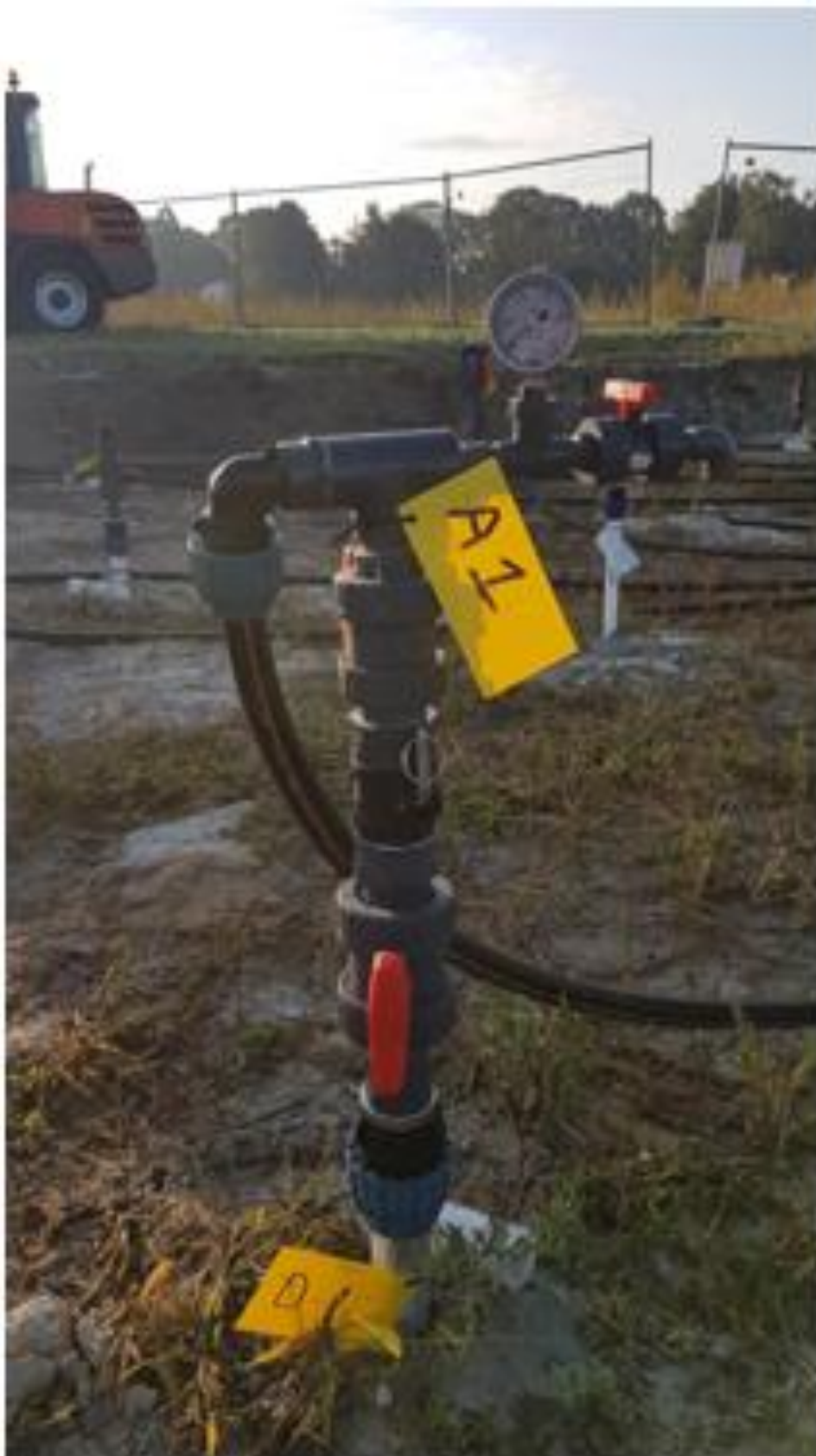
Detail injection well manifold
