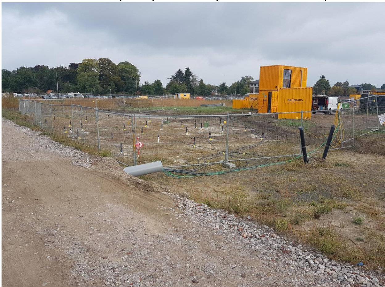
Overview injection filters in source zone
