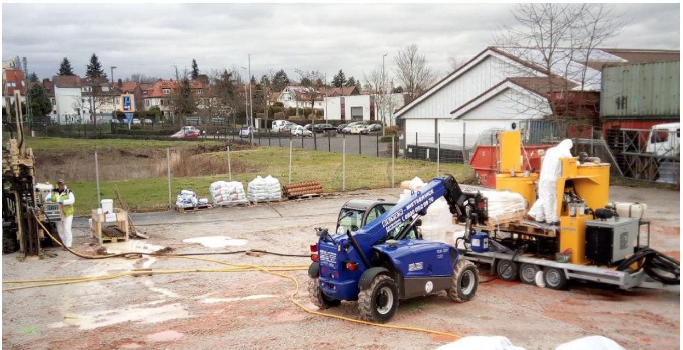
High pressure injection/fracturing/ and mixing equipment used for fracture-emplacement of persulfate-peroxide oxidant slurry into subsoils through direct push drill holes
