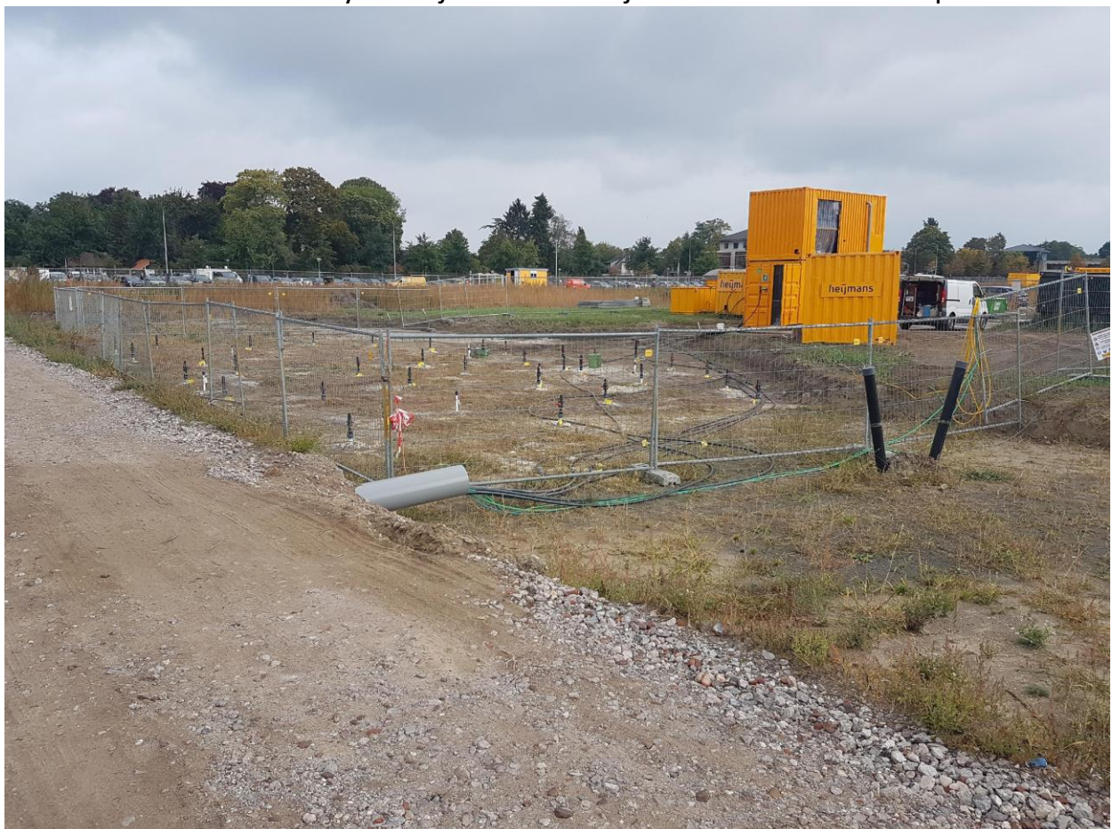
Overview injection filters in source zone
