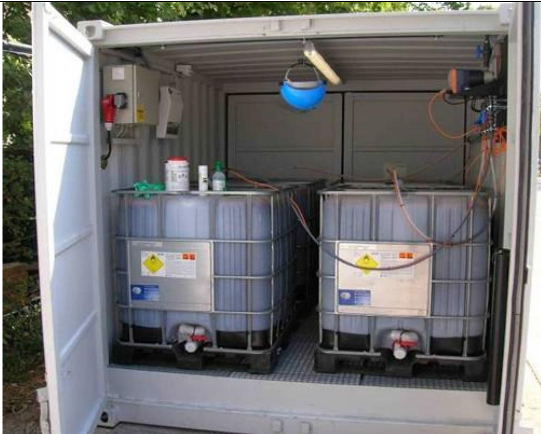
ISCO dosing station
