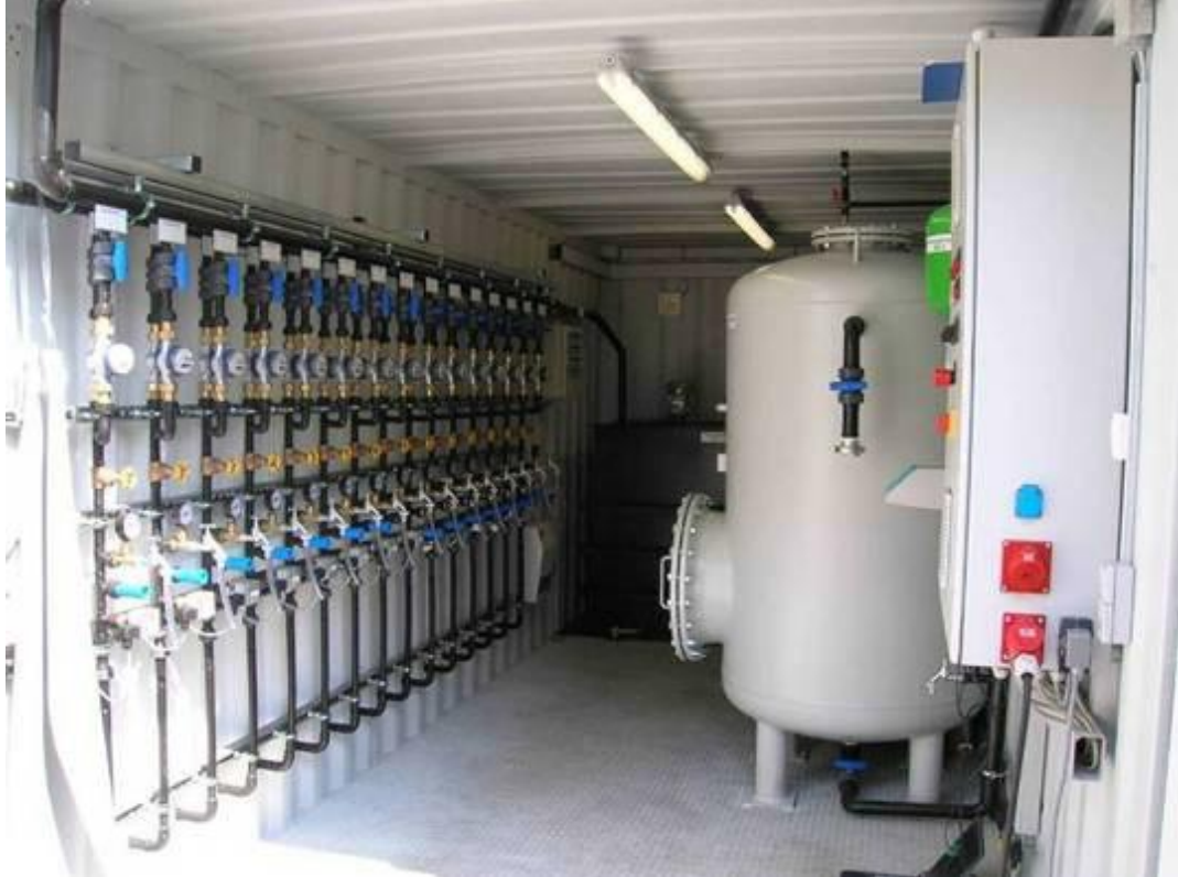
ISCO plant technology
