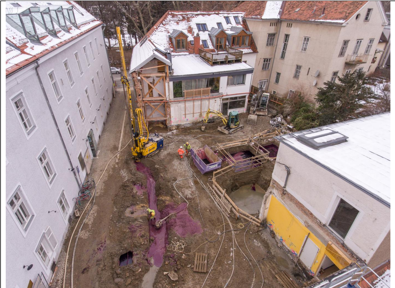
A picture of the site. Works are conducted below former washing machines. Backflow deeply covered purple by \text{KMnO}_4
