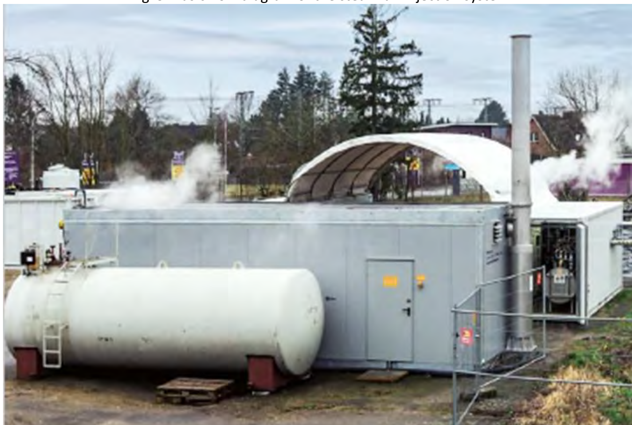
Fig. 10: Container with steam generator unit and fuel oil tank
