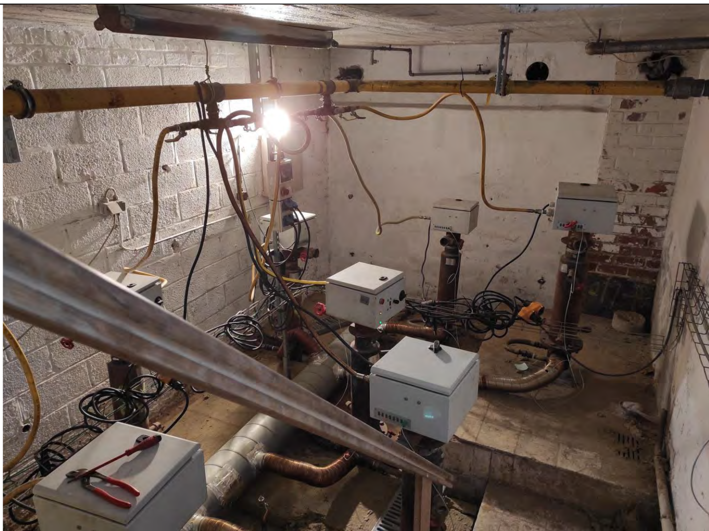
Figure 4 - Treatment Zone 2 in the basement
