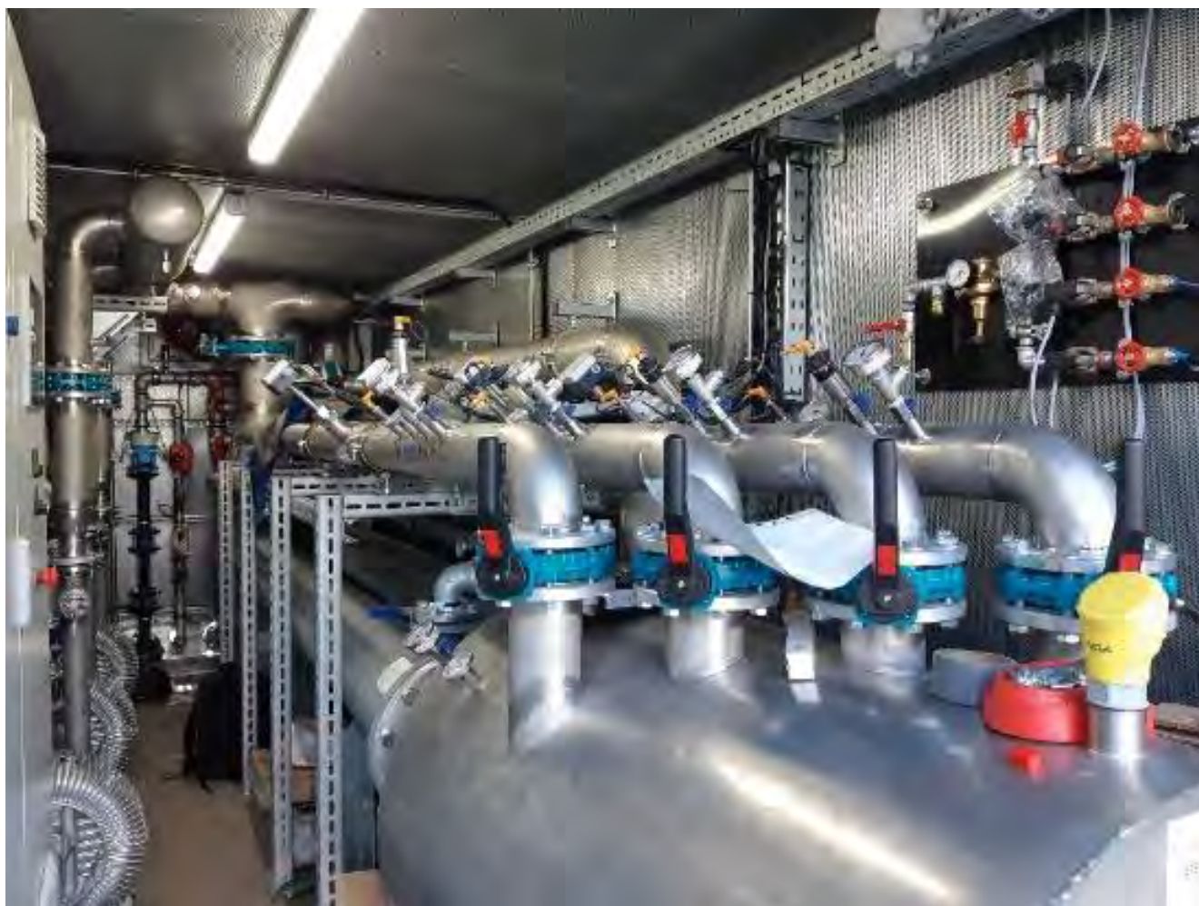
Fig. 12: Raw air measuring sections and condensate separator of the soil vapour extraction system
