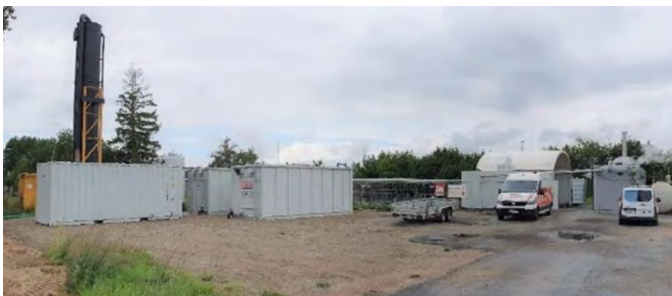
Fig. 13: Remediation system with groundwater purification plant (left side)
