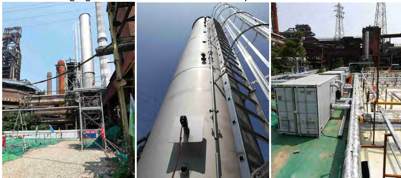
Figure 11 – 12 – 13 - Treatment plants (flare stack, SVE-plants)
