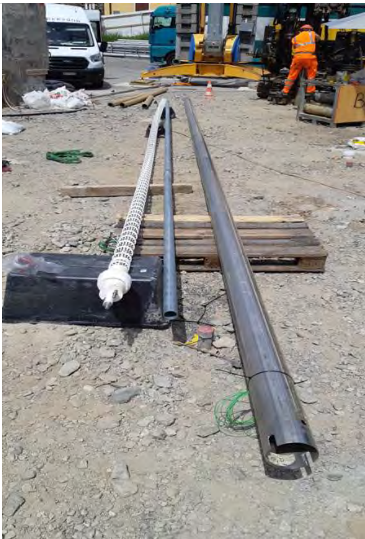
Figure 12 - Electric heating element (HEL) of 8 m length (left) and a protective tube (right)
