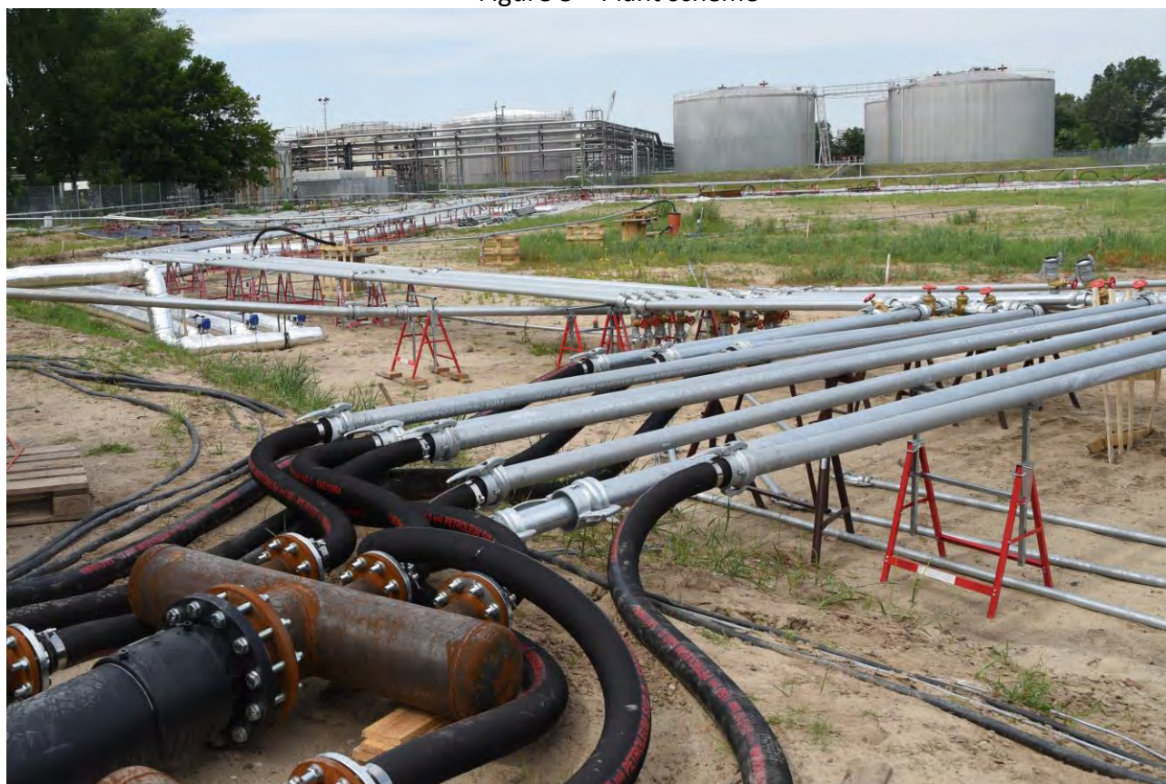
Figure 9 – SVE-pipes from the field
