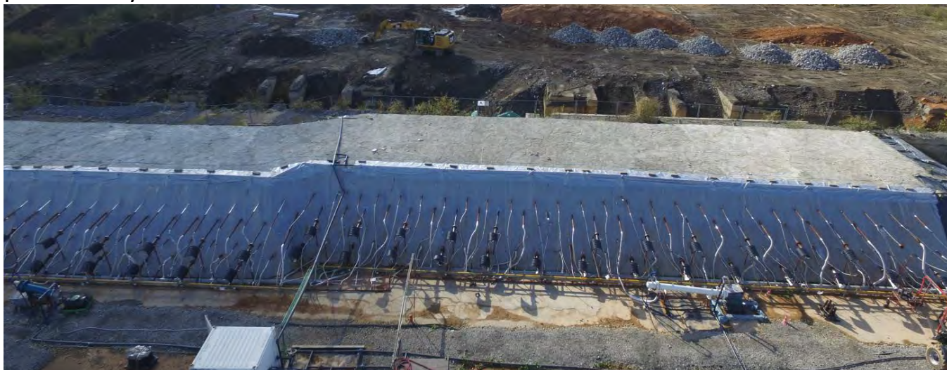
Figure 7 – Main treatment unit (picture)
