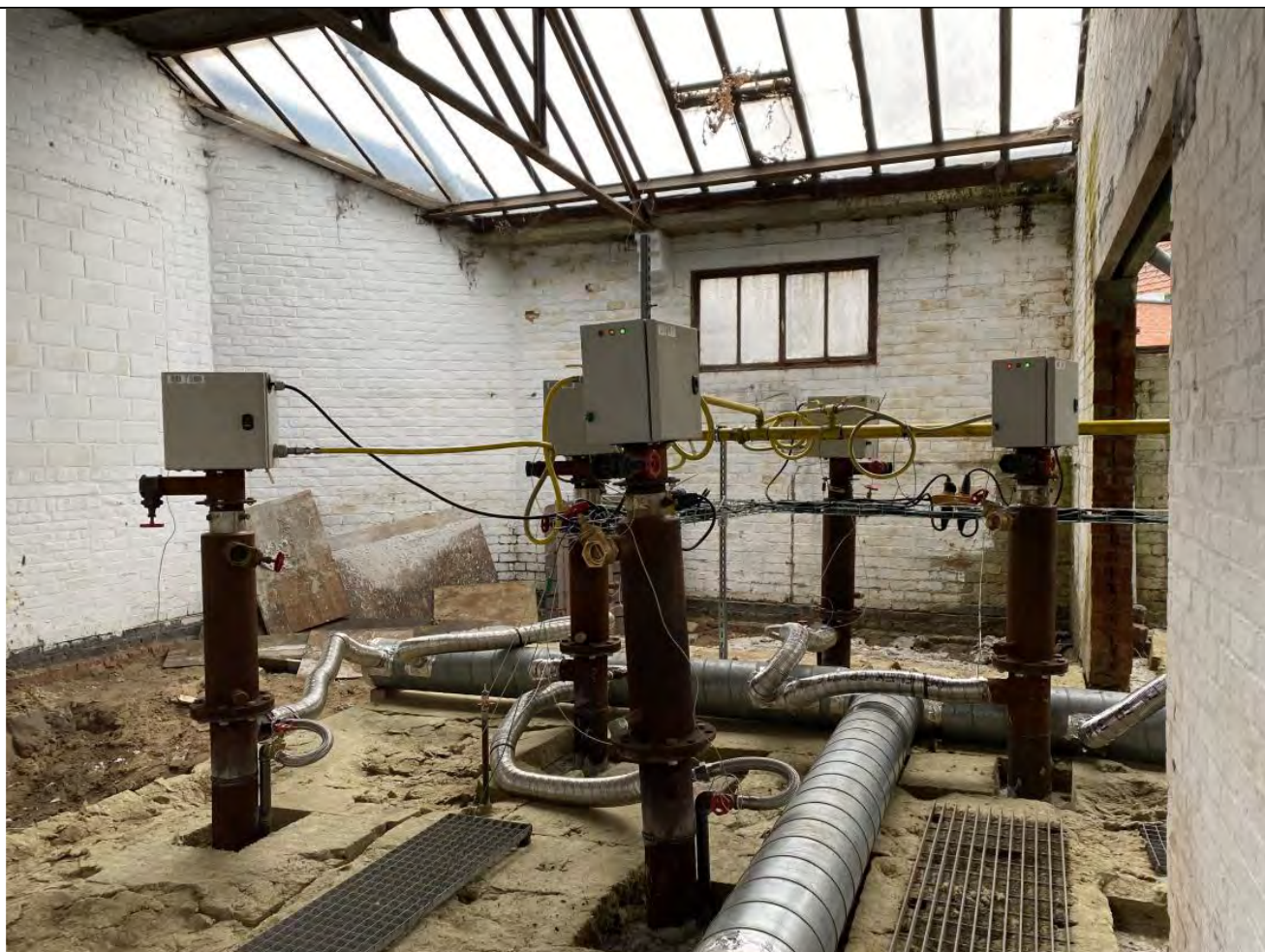
Figure 2 – Back area of the site with its Smart Burners™
