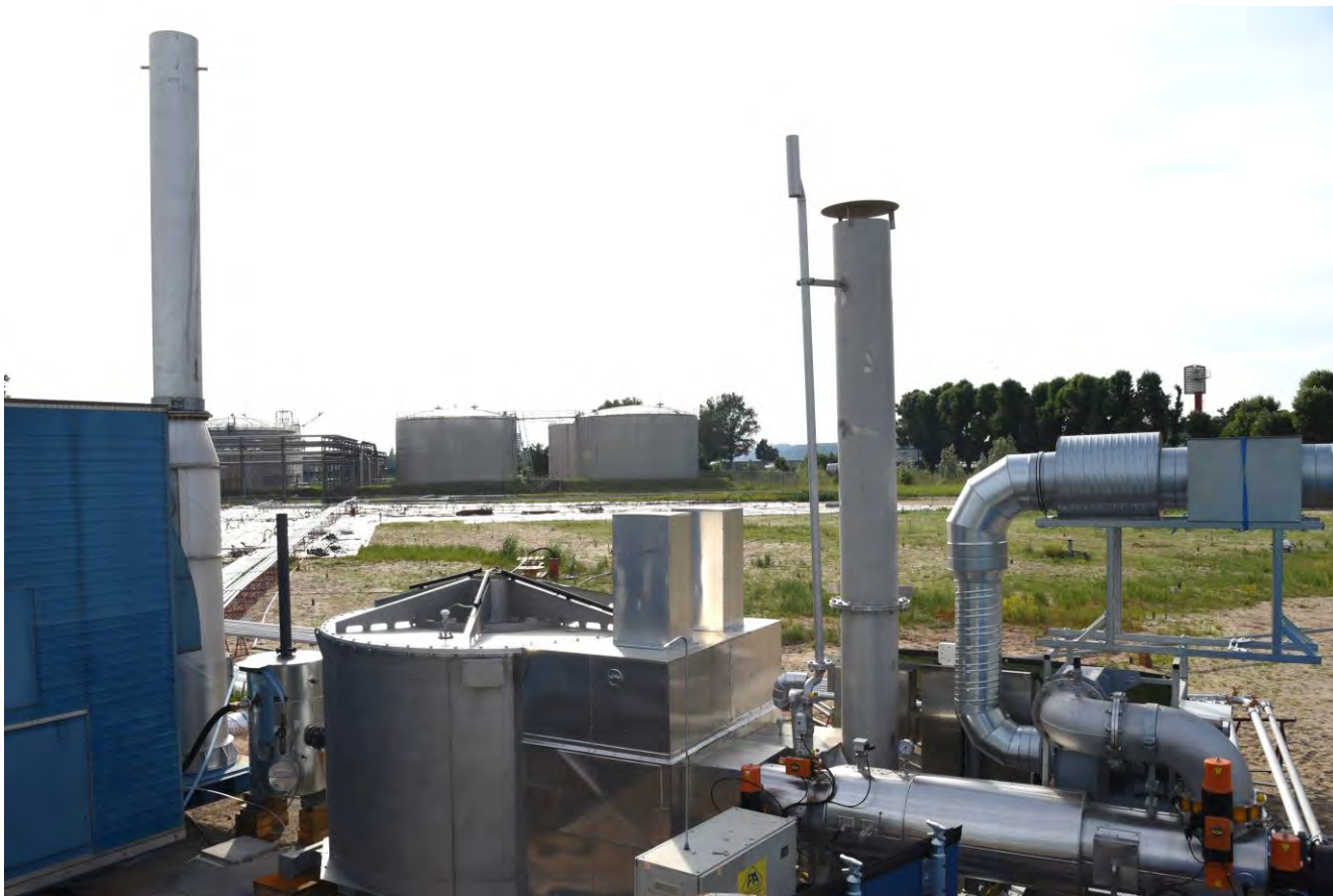
Figure 13 – Steam boiler (left), RTO (right), remediation field
