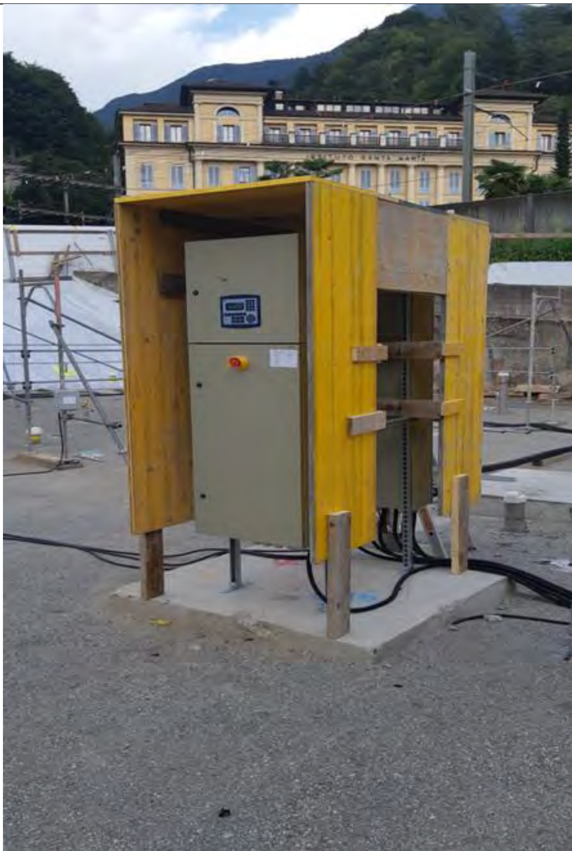
Figure 13 - Control cabinet in the field
