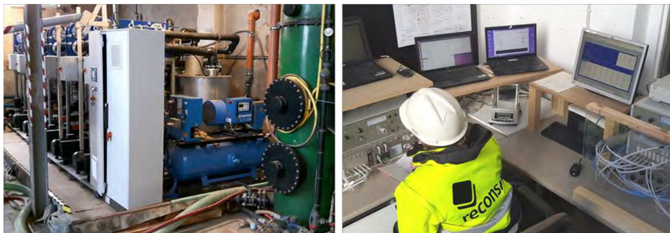
Figure 8 – Heating and remote control room
