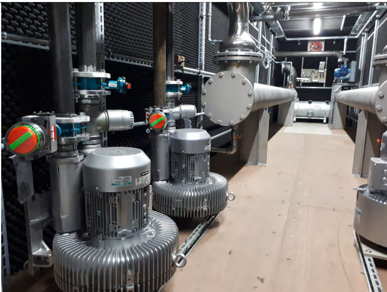
Figure 13 - Extraction fan (foreground) and air/water heat exchanger in the background
