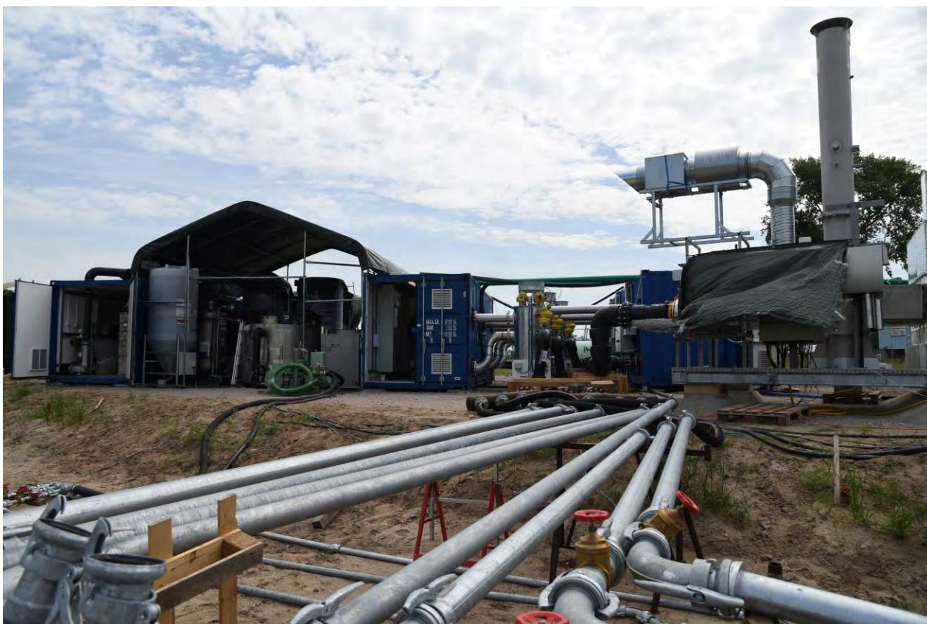
Figure 12 – Water treatment (left), RTO (right)
