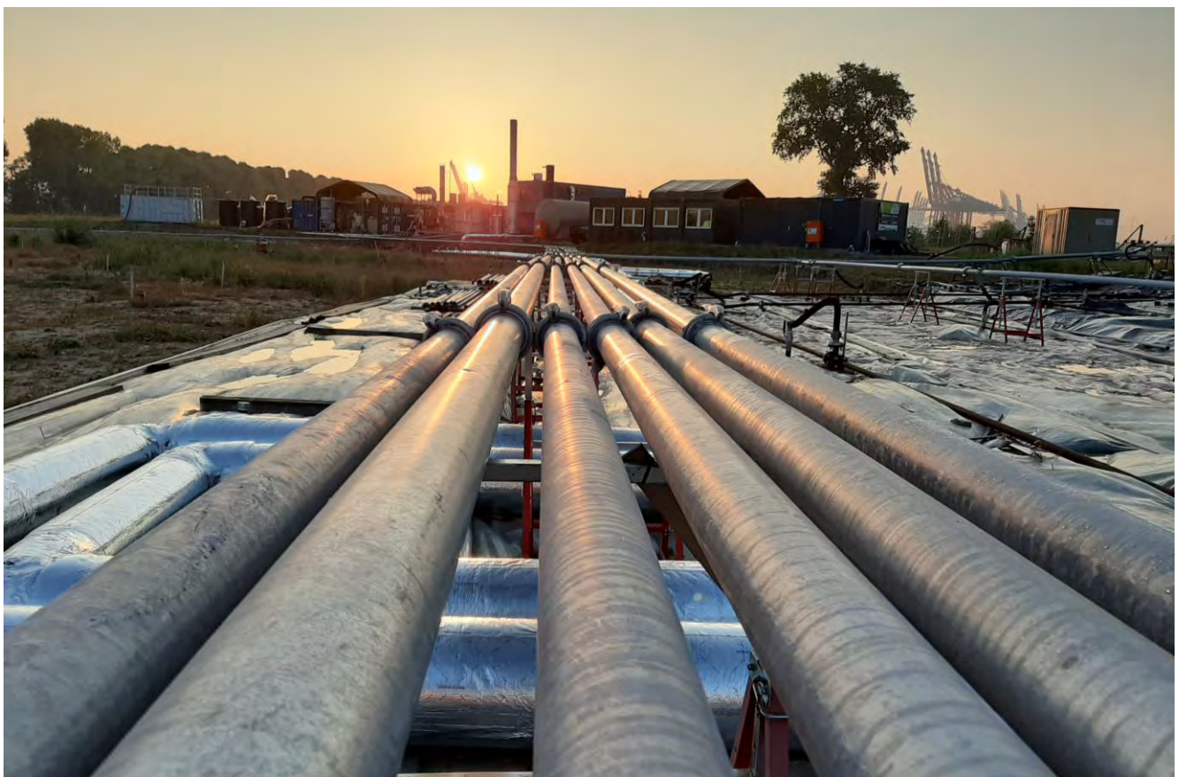
Figure 10 – SVE-pipes from the field to the treatment plant
