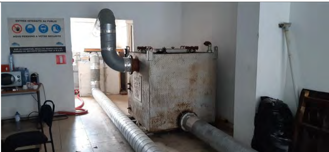
Figure 2 - Activated carbon tank
