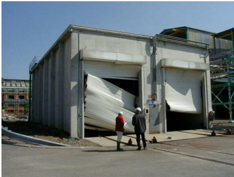
Building housing the chlorine stocks and tankers
