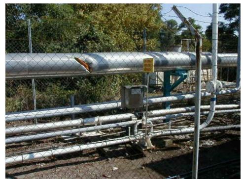
Impact made by flying debris on a water pipe
