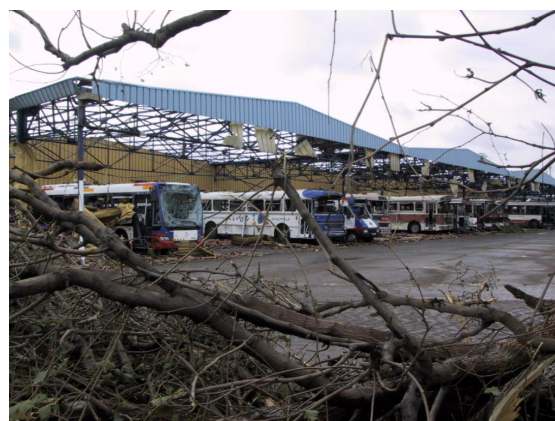
Bus depot destroyed
