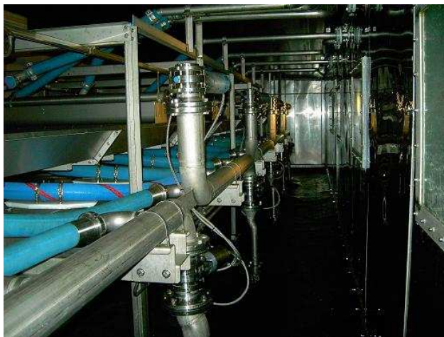
View of the filter inside the enclosure (RR)
