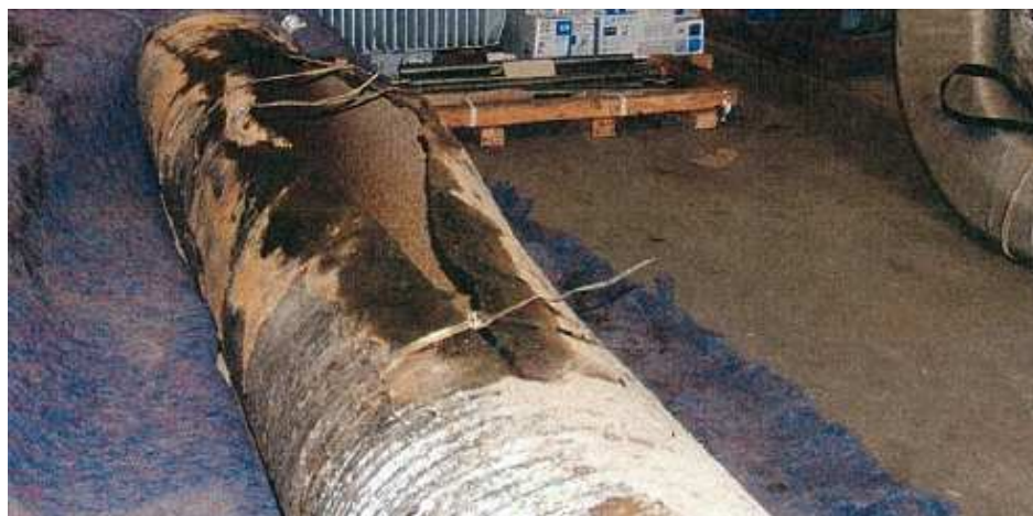
Damaged part (DREAL PACA)
