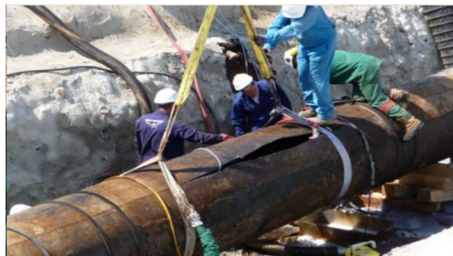
"Button-hole" opening of the 40-inch pipeline (RR)
