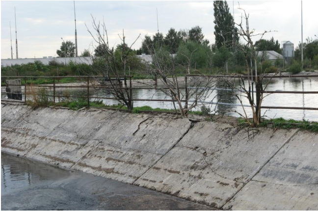
Technical state of the slurry tanks
