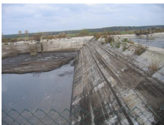
Technical state of the slurry tanks
