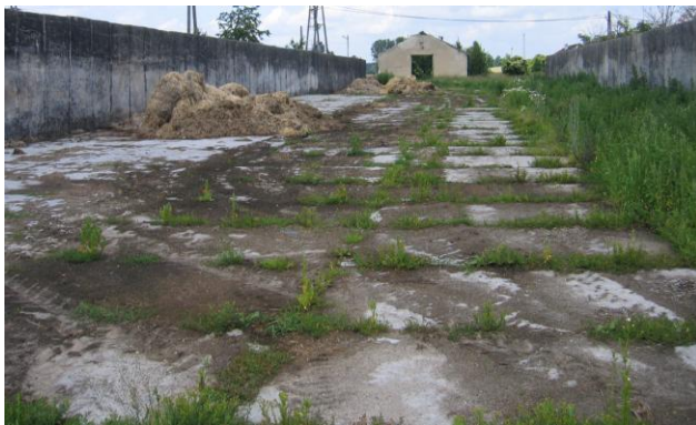
Damaged dung slab
