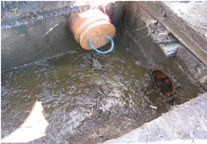
Yard drainage diverter system
