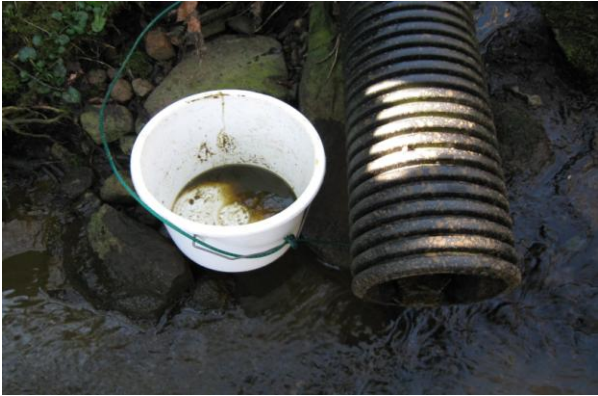
Discharge to water course
