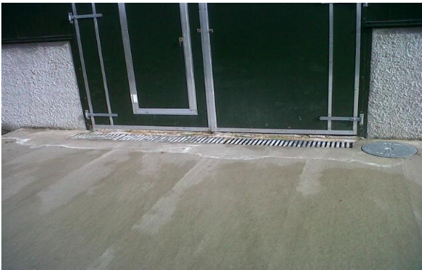
House washings. Routing directly to storage tanks
