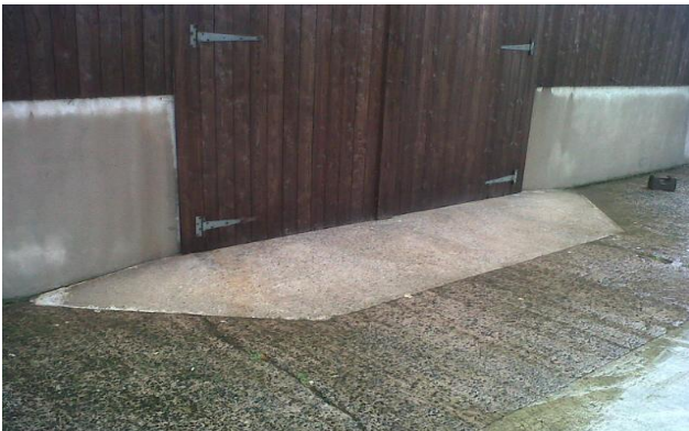
House washings. Reliance on yard drainage diverter
