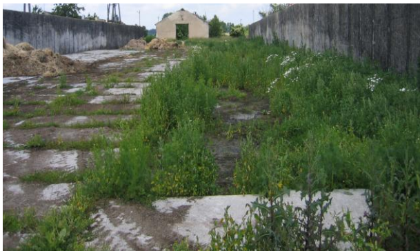
Damaged dung slab
