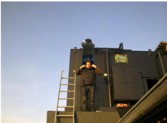
Inspection air scrubber
