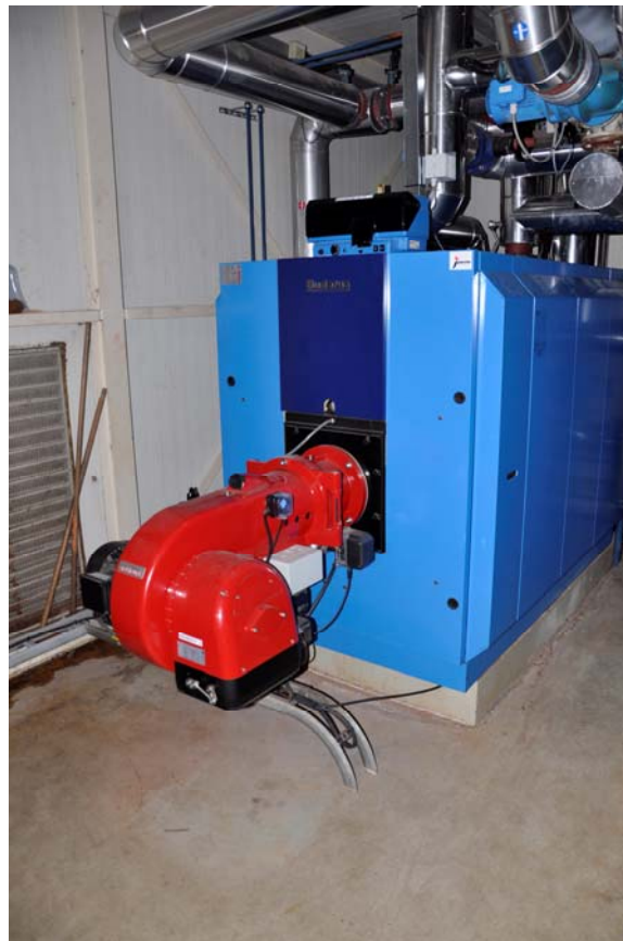
Fig. 11: Boilers fired on biogas
