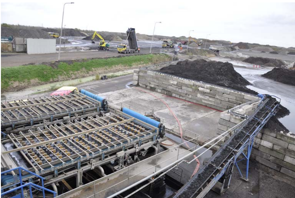
Fig. 14: Soil treatment facility
