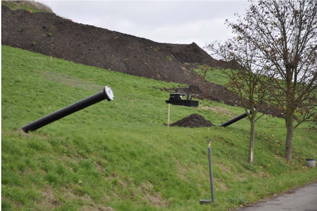
Fig. 7: Piping and well of the leachate-system
