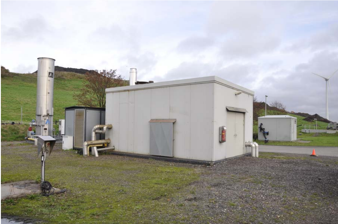
Fig.10: Biogas extraction unit and flare
