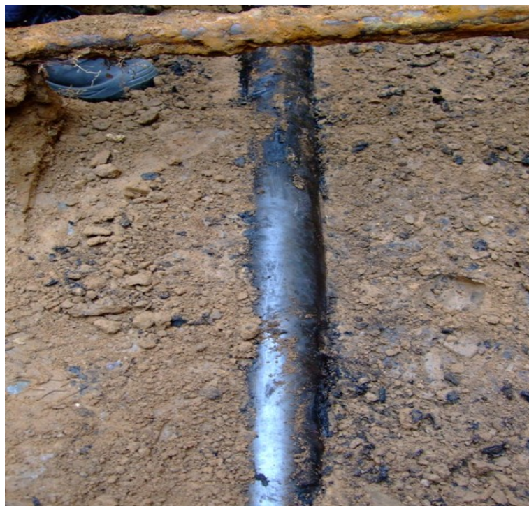
Figure 4: Water pipe (at the top of the picture) crossing the kerosene pipeline (copyright: operator)
