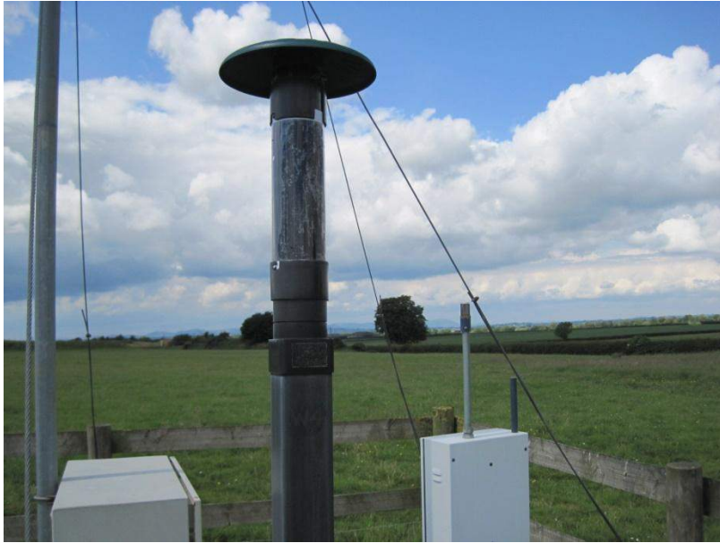
Fig. 13: Dust monitoring installation
