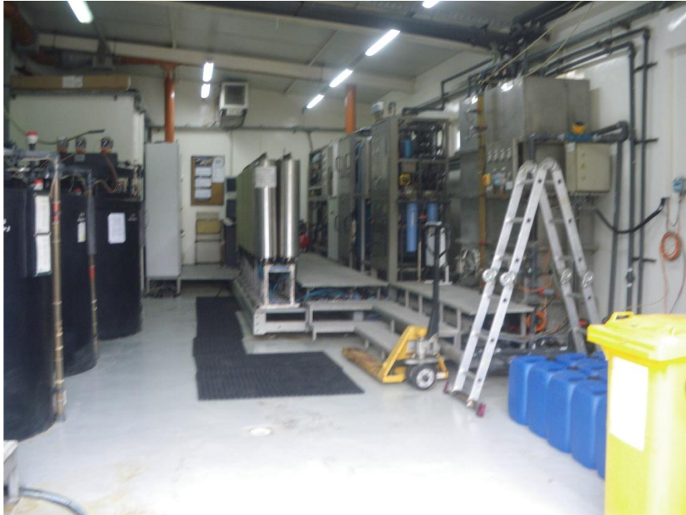
Leach ate treatment plant
