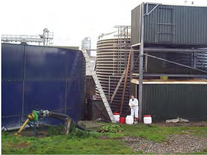
Figure 1-3: Example of a 335 m 3 capacity digester [Figure 4.56; IRPP BREF Draft 1, 2011]
