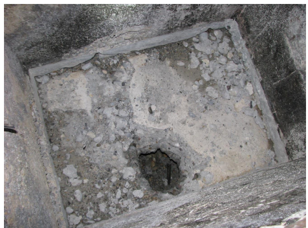
Hole in the floor of the chemical effluent shaft (close-up) © Site operator
