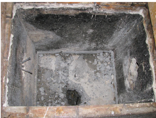
Damaged chemical effluent shaft © Site operator
