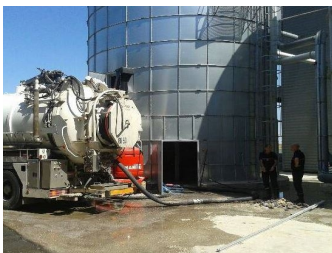
Drainage of the silo © Fire Services
