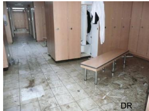
Changing rooms after flood
