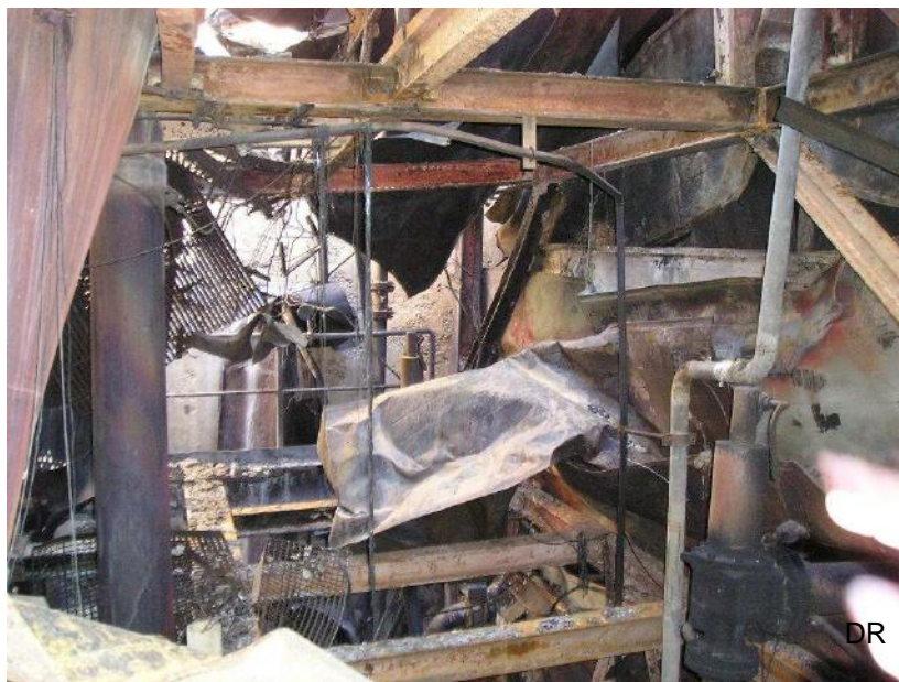
The destroyed "cold box"
