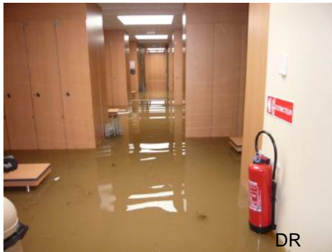
Changing rooms during flood
