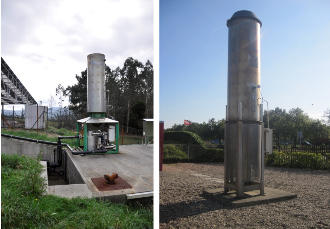
Figure 17: Landfill gas flares examples
