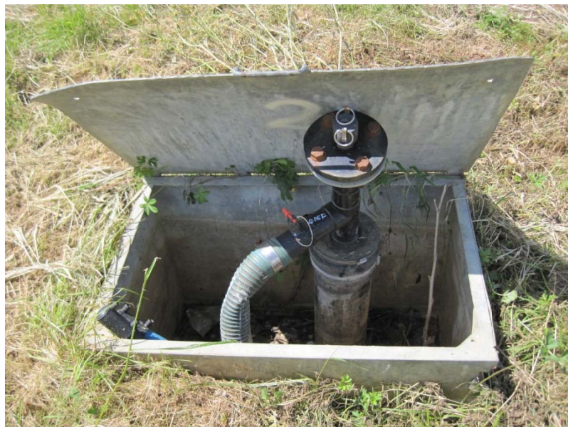
Figure 15: Landfill gas collection boreholes
