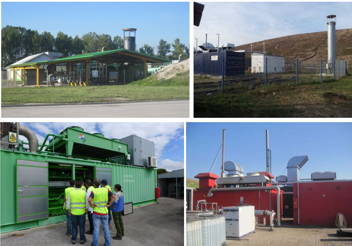
Figure 19: Energy power plants
