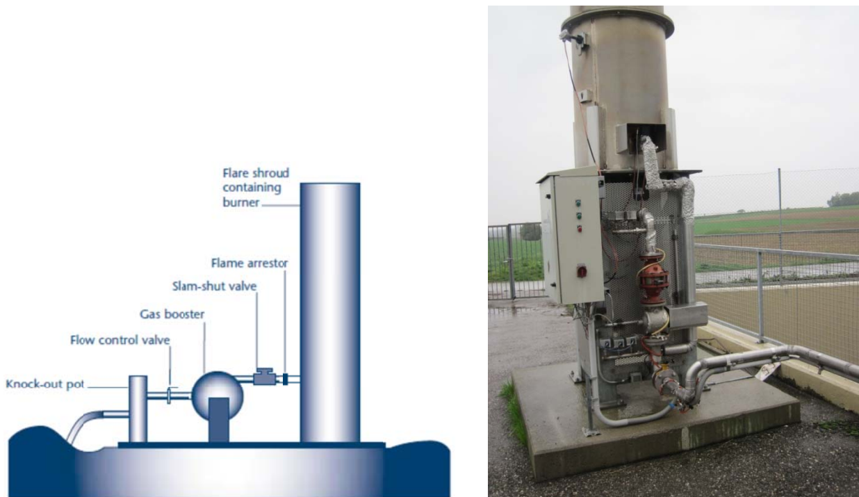
Figure 16: Landfill gas flare
