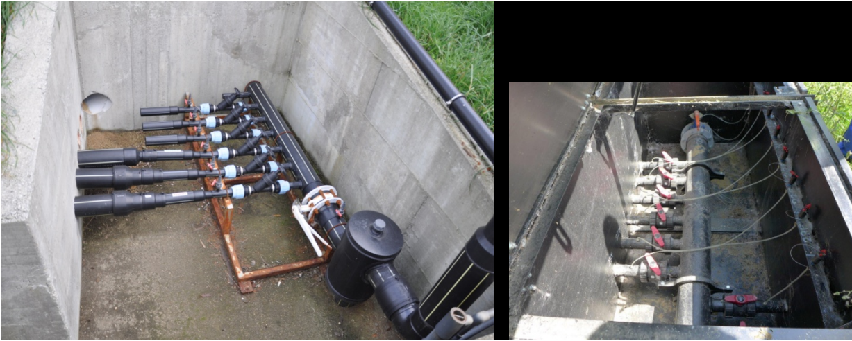
Figure 10: Landfill gas piping
